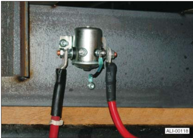
Power cut-off solenoid.
